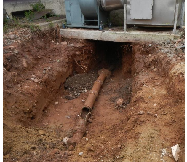
Evidence of the problem
