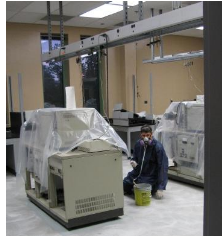
Mariusz dons protective equipment while coating the floors with an epoxy finish.
